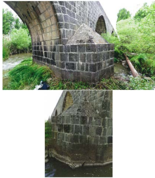
Figure 13. Corrosion of the pier due to the presence of water
