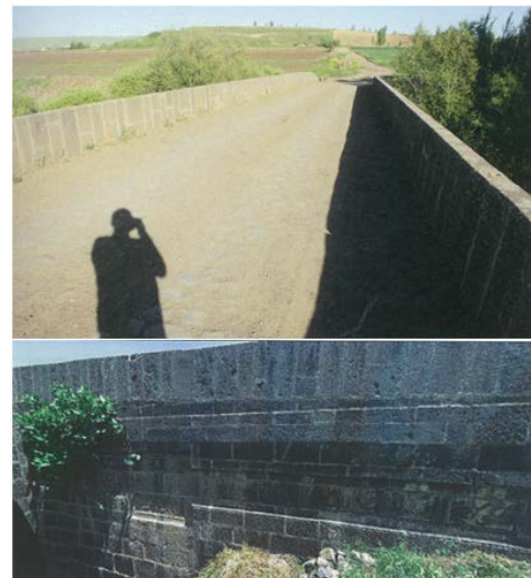
Figure 15. presence of vegetation on roadway and spandrel walls
