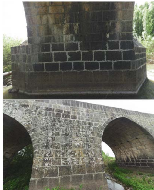
Figure 14. presence of fungus on the stone surfaces
