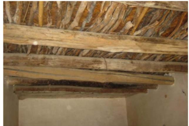
Figure 7. Wooden beams used in the ceiling in historical houses in Erbil ( http://www.erbilcitadel.org/ )
