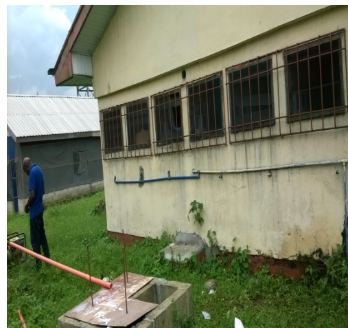
Figure 4. Preparing the feed line for the delivery of the septic waste into the anode chambers
