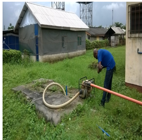
Figure 3. Connecting a generator to the septic waste at the female hostel
