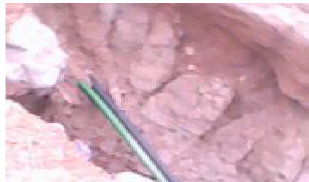
Figure 3. Exposure of utility cable by gully erosion, Minna, Niger State of Nigeria (Personal photo taken by the leading author, 2012)
