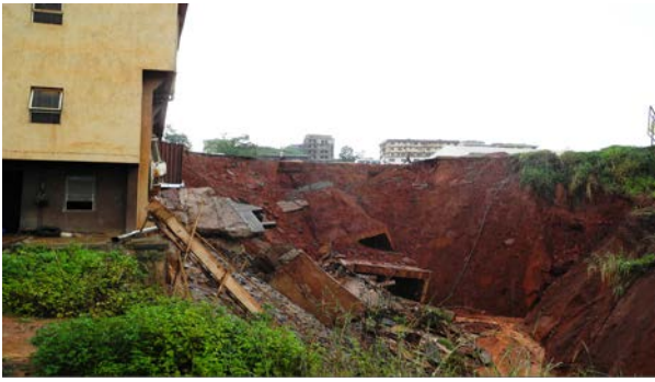
Figure 5. A three-storey building about to be swallowed by gully erosion at Omabge Estate, Onitsha (News Agency of Nigeria, 2011)
