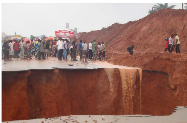
Figure 6. Road hazard resulting from gully erosion at Orlu/Mgbee road (imostateblog, 2012)
