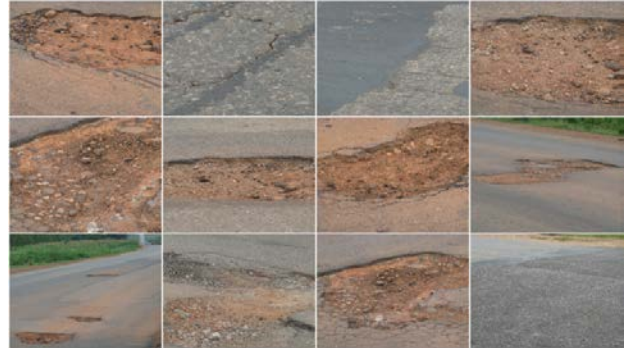
Figure 3. Sections of Minna-Bida road showing potholes, failed spots and uneven road surfaces (Courtesy: Authors, 2013)
