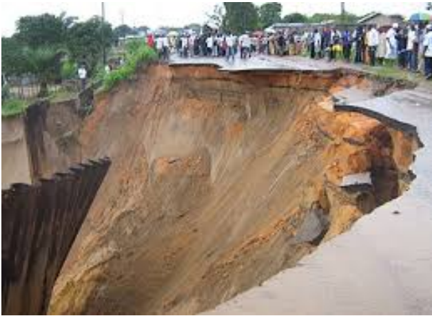
Figure 2. Landslide along a major roadway in a District in Brazzaville
