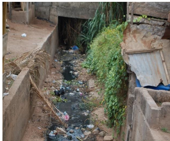
Figure 1. Solid waste dumped in open storm drains (Source: (Fieldwork, February, 2020))
