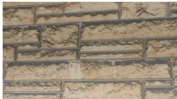
Figure 2. Lattimer building stone façade with thick accumulation of black dust
