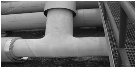
Figure 2. T-tube on the pipe
