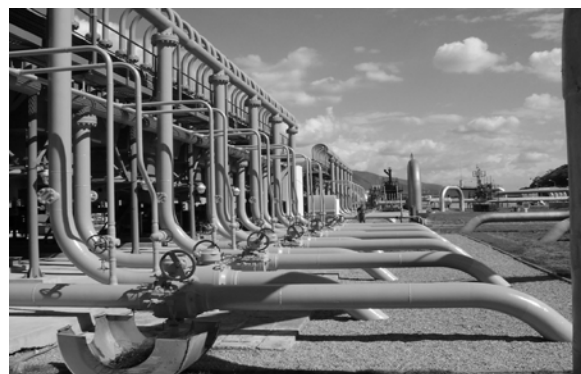
Figure 1. Pipe yard of compressor station
