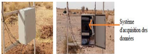
Figure 4. Measurement device and data acquisition system installed
